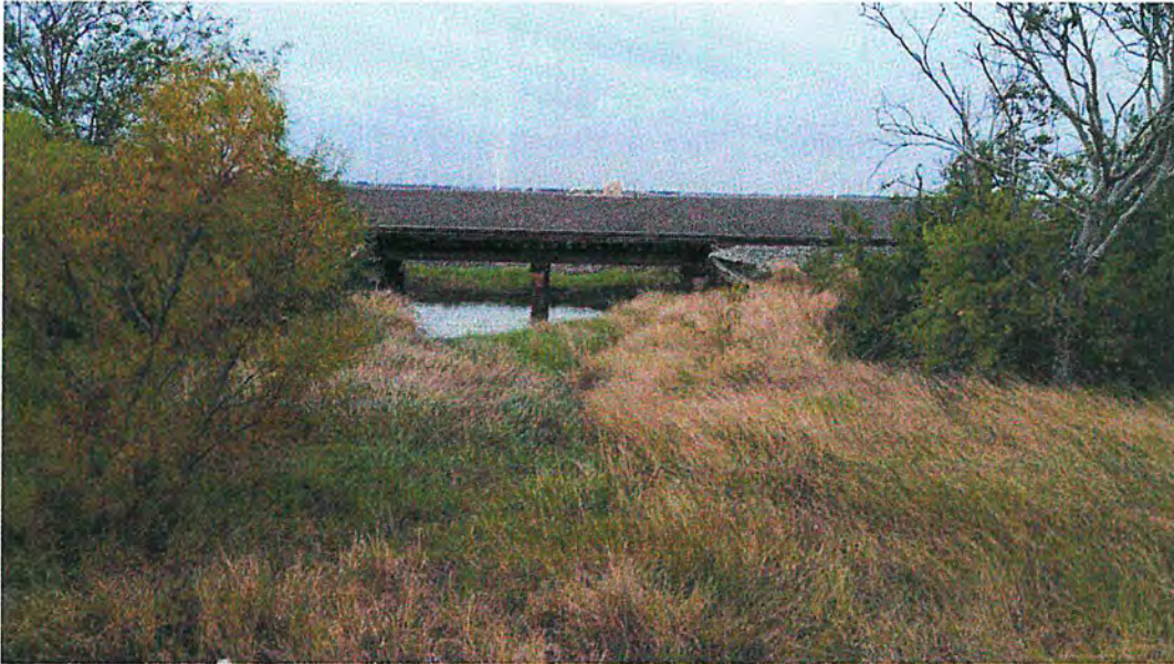
5. Outfall 003 proposed location, looking south (upstream). Railroad track in middle of photo. Drainage channel center, in front of track.
