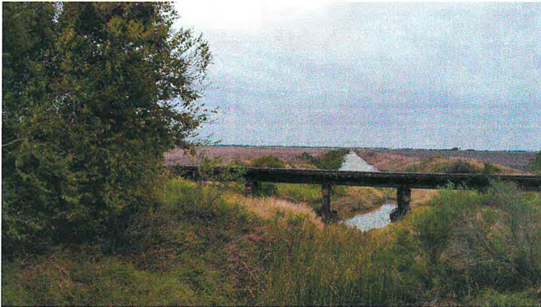
3. Outfall 002 proposed location, looking south (upstream). Railroad track in middle of photo. Drainage channel center.
